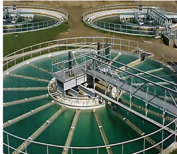
3.3.6 Water Purification centre
