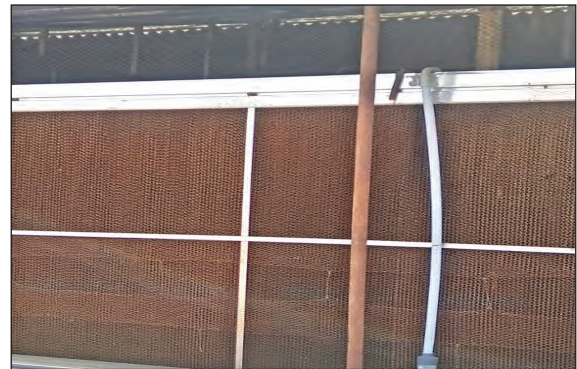
House with cooling pads
