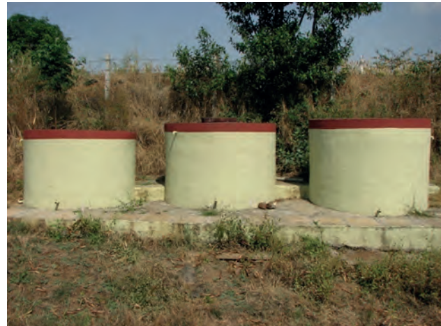
Rainwater harvesting tanks
