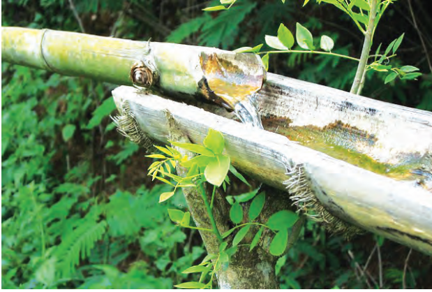
Figure 5.5 : Bamboo Irrigation System
